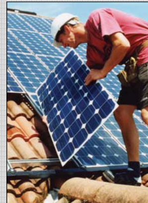
Roof mounted PV array
